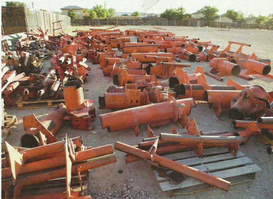
REST IN PIECES: Using the Spectrum 1000, each section of the High Roller track took about three minutes to cut. Using oxy-fuel would take seven minutes for each section. With about 367 sections, the time difference is 19 vs. 43 hours of cutting time.
