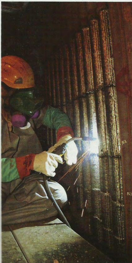
Fig. 5 — Welders become productive more quickly with the newer pulsed equipment because setup is quicker, less complicated, and requires less training, noted Brad Hooper, supervisor, Northeast Regional Maintenance, Covanta Energy.
